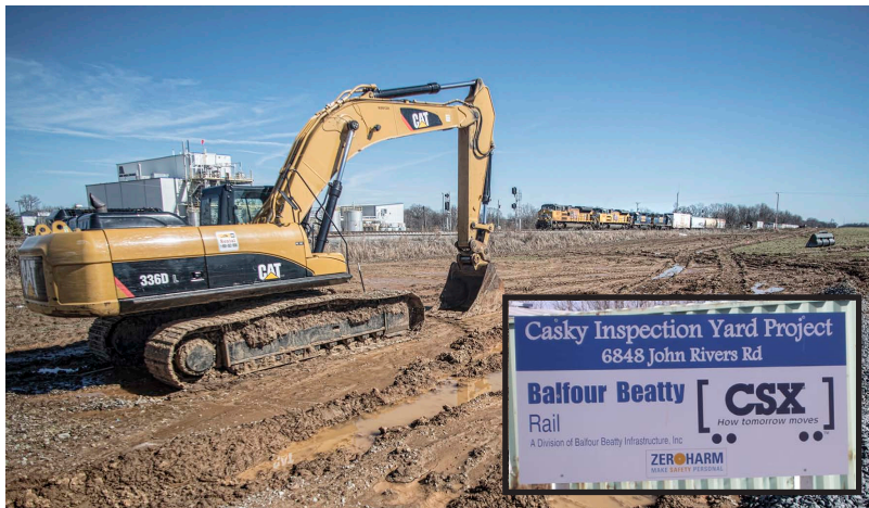
Above: On February 22, 2014 a northbound CSX mixed freight, headed up by two UP engines, heads past the area where the new south lead will be for the new Casky Yards on the Henderson Subdivision will be located on John Rivers Road, south of Hopkinsville, Ky. Some construction has begun, but with the wet weather we've been having lately much of the dirt and track work has kept the equipment building the yard idle. -Jim Pearson
